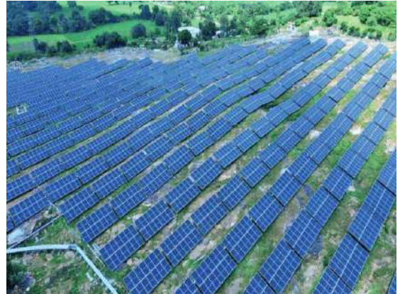
Figure 14.1 SANCHI - SOLAR FARM
